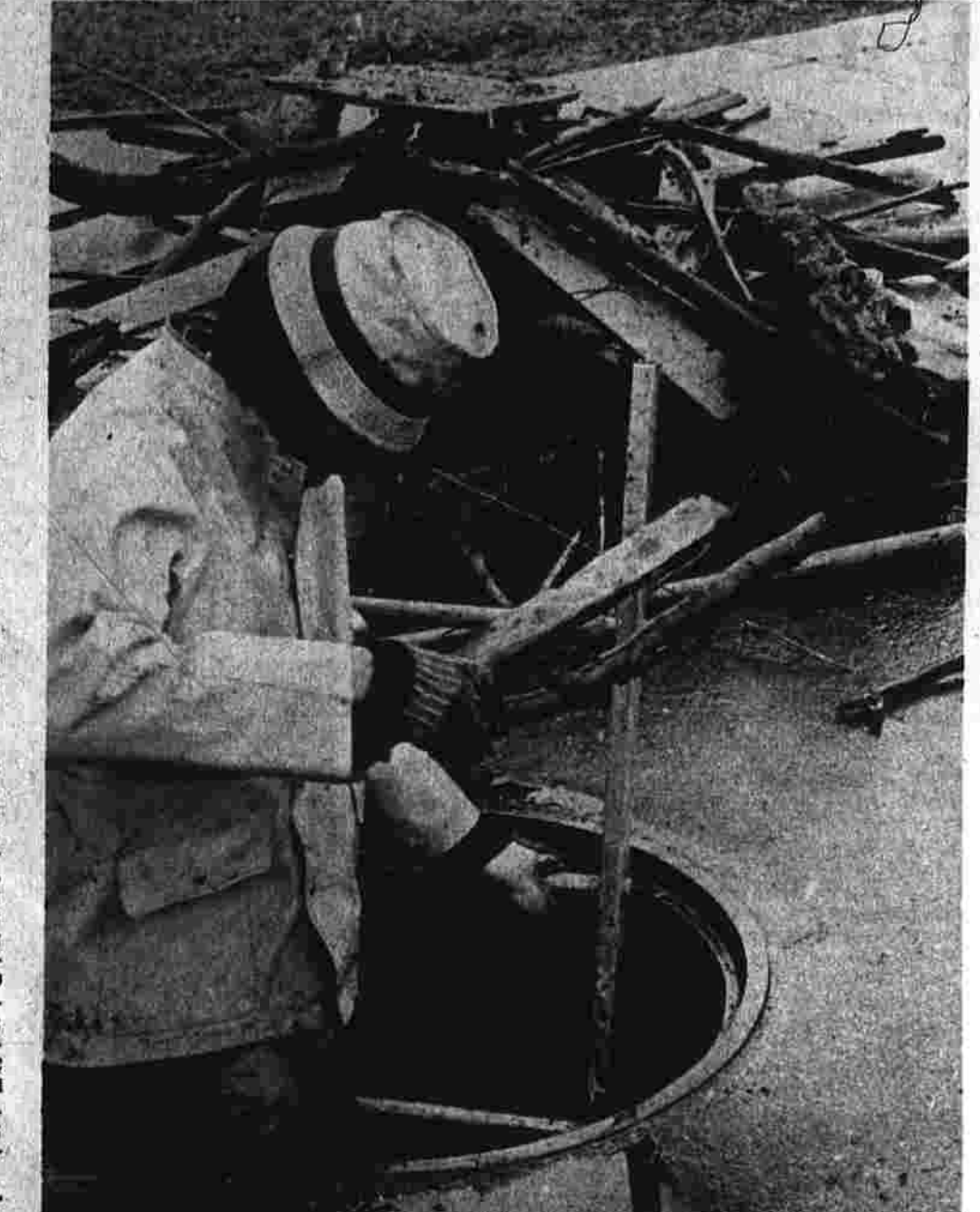
This pile of debris was cleaned Thursday from a catch basin at N. Main and Oakland Sts. On the ladder and getting the last of it is an employee of the Manchester Public Works Department.
